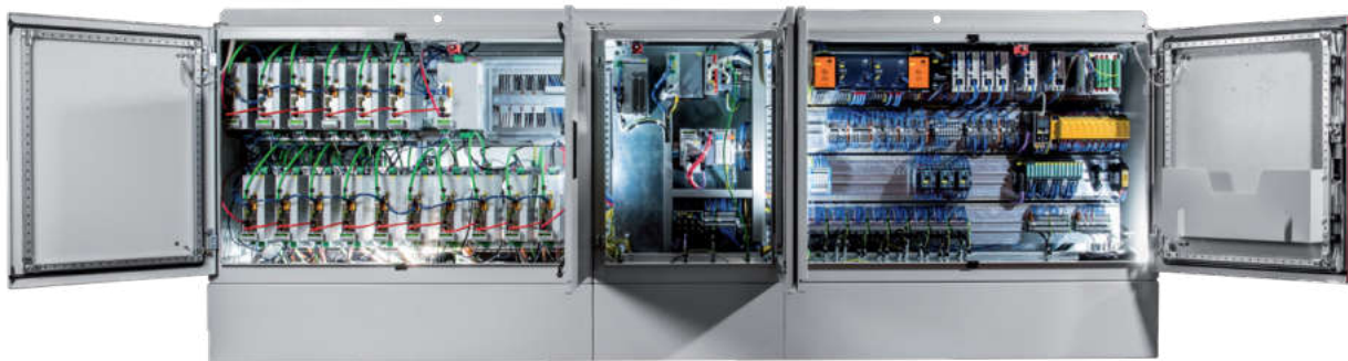
A look at the new compact control cabinet
